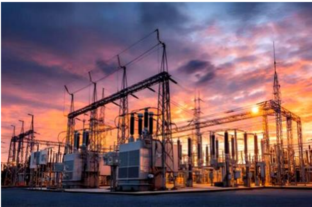
Electrical Substation—Source: Vecteezy, 2026
