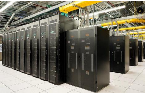
Server Halls/Racks—Source: Maheswari Sushant, Aug 27, 2023
