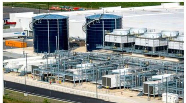
Above-ground water storage tanks and cooling towers— Source: Yancey Dwayne, February 9, 2026
