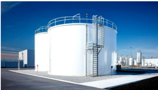
Above-ground gas storage tanks—Source: LUTZ, 2026
