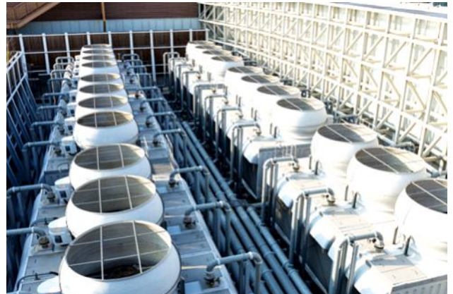
Cooling Towers/Water Treatment—Source: SAMCO, 2026
