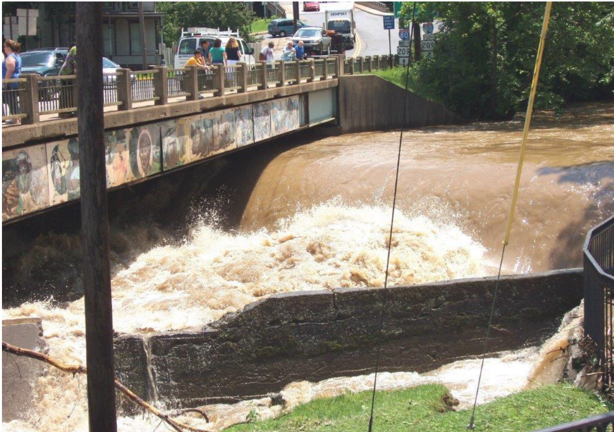
Figure 22 - A Flooded Stream Flows Under a Monroe County Bridge
