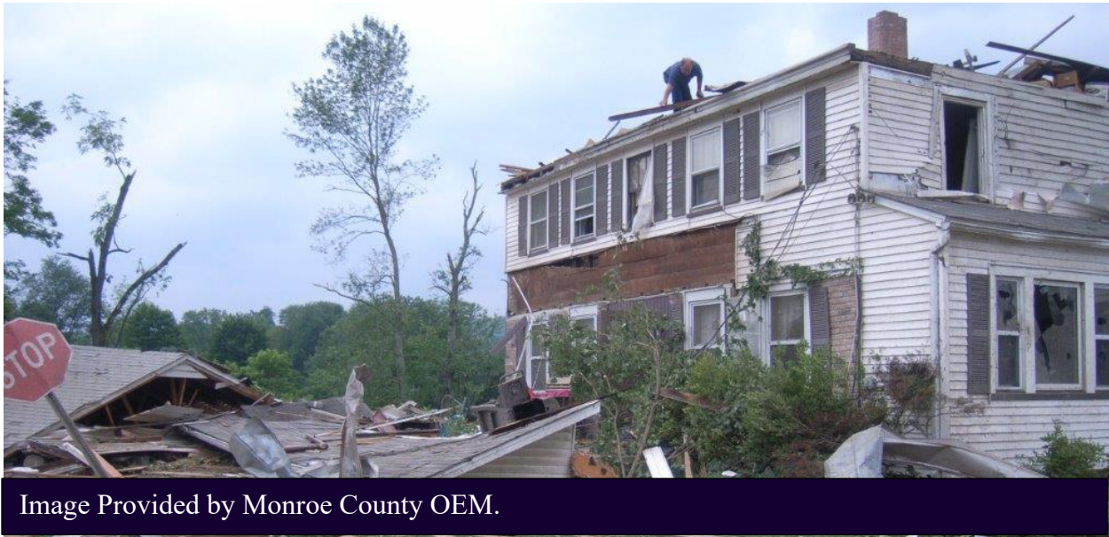
Figure 34 - Property Damage is Assessed Following a Tornado
